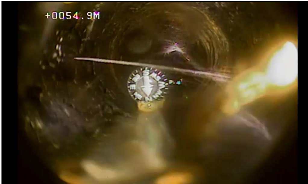
Figure 1: CCTV Screenshot - Seepage
