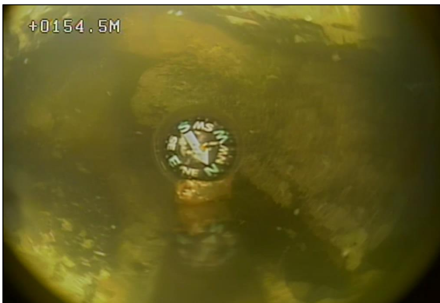
Figure 2: CCTV Screenshot - Blocky rubble
